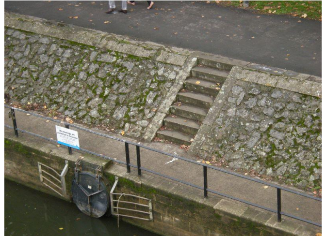
Photo 6: Steps down bunded slope have no handrails
