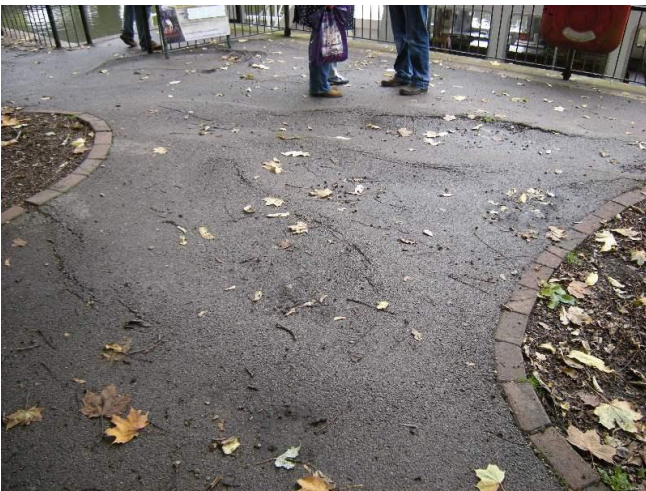
Photo 15: Uneven tarmac is a potential trip hazard
